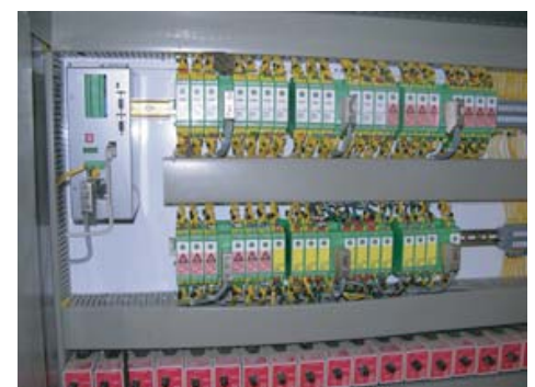
The Controlstar® and I/O
