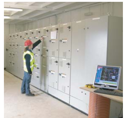
Panel and local SCADA
